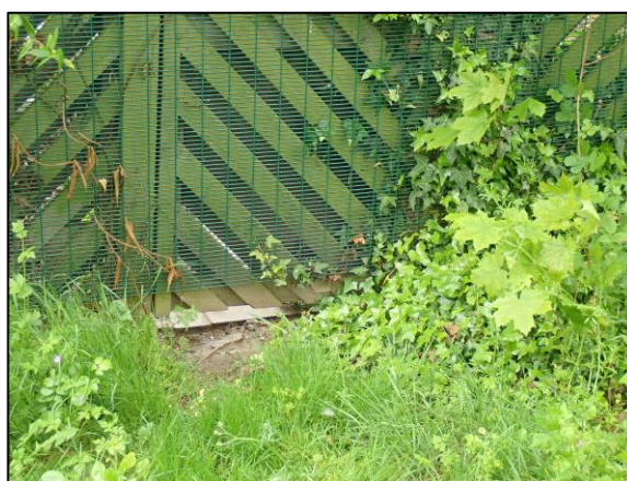
Photo 10 Push-under beneath rear fence
