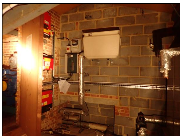
Photo 11 Internals of service area in Loft 1
