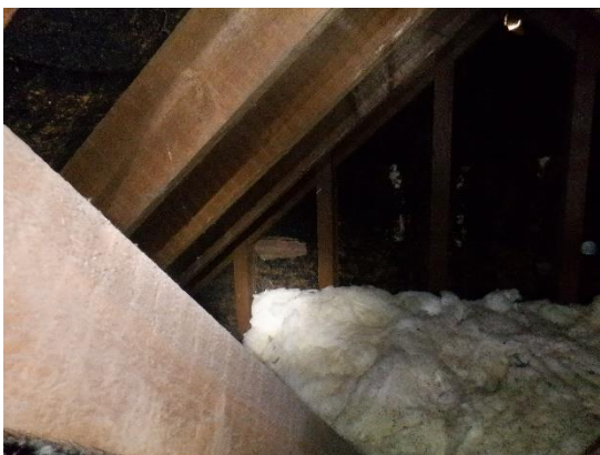
13. Tear in bitumen felt on front (roof void).
