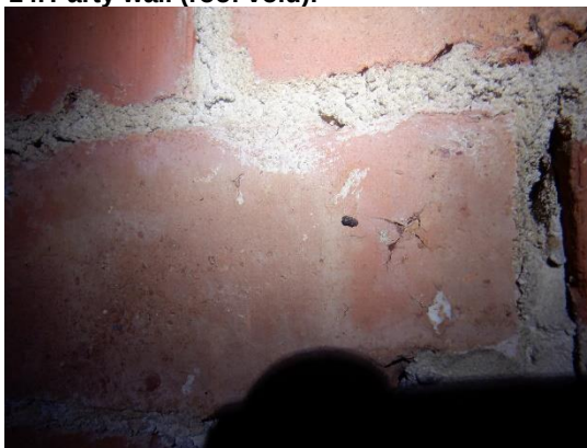
16. Small bat dropping on party wall brickwork (roof void).
