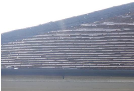
4. Missing mortar below hip tiles (rear elevation).
