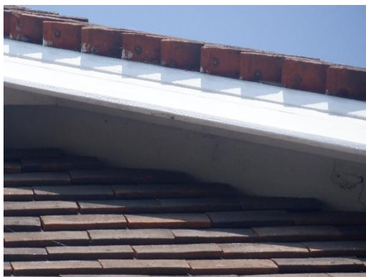
7. Gaps over hanging tiles beneath gable soffit (front elevation).
