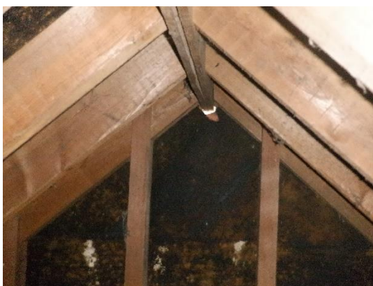
12. Daylight visible through gap at apex of front gable (roof void).
