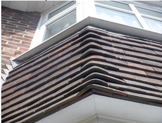
6. Lifted hanging tiles above bay window (front elevation).
