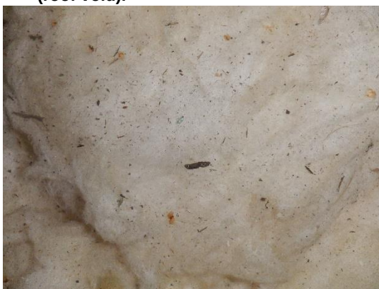
18. Medium-sized dropping on fibreglass insulation (roof void).
