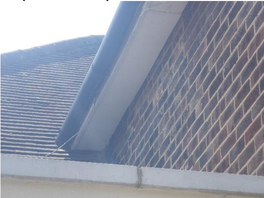
5. Slight gap between soffit and brickwork (side elevation).
