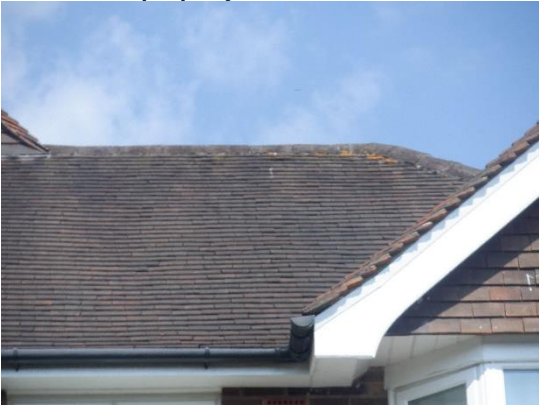
3. Occasionally lifted overlapping roof tiles (front elevation).
