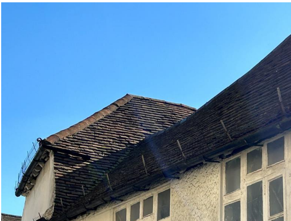
Photograph 35: Main Pub, gaps at eave and missing tiles, eastern elevation
