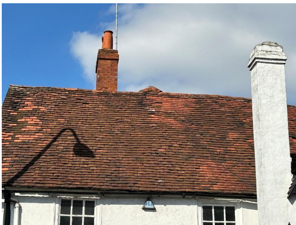
Photograph 31: Main Pub, lifted and slipped tiles, southern elevation
