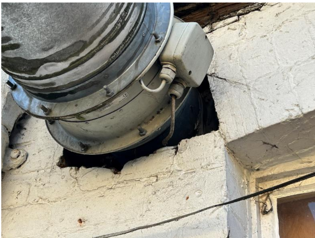
Photograph 43: Barn, holes in masonry, eastern elevation
