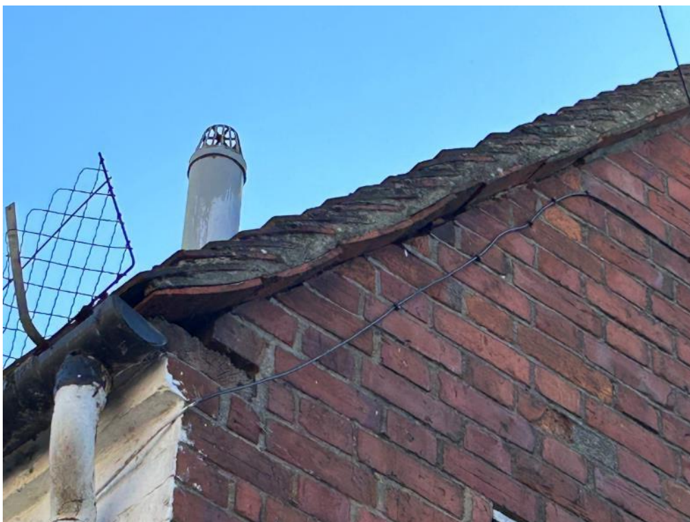
Photograph 37: Main Pub, eaves overhanging Barn, gaps leading into roof
