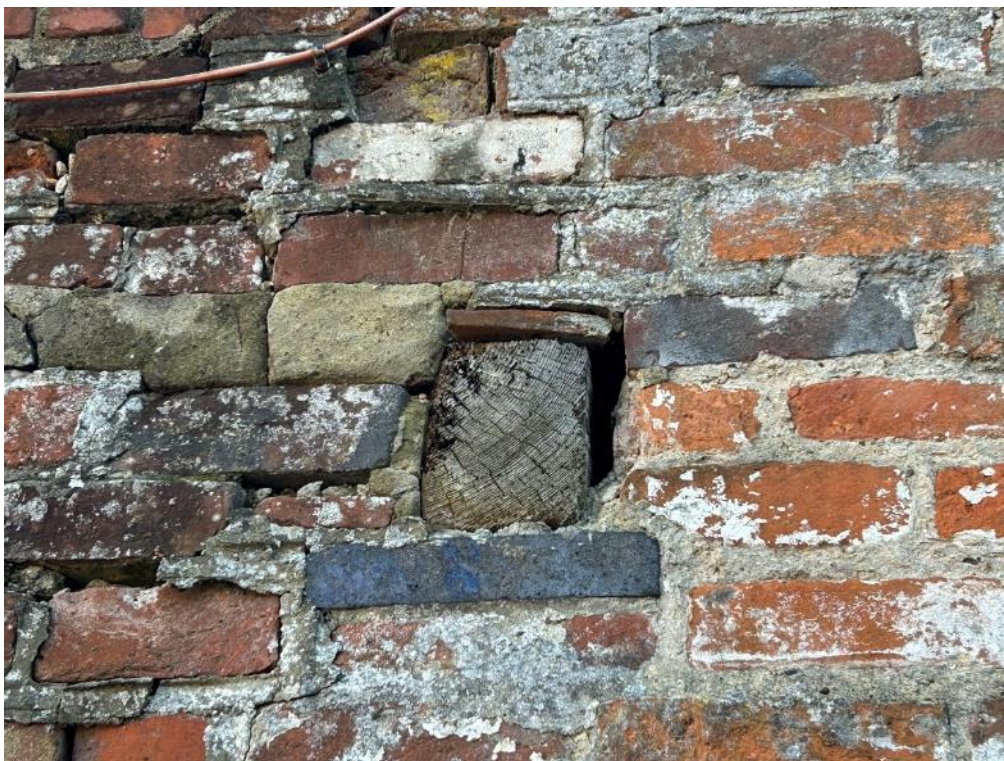
Photograph 42: Barn, holes in masonry, northern gable end
