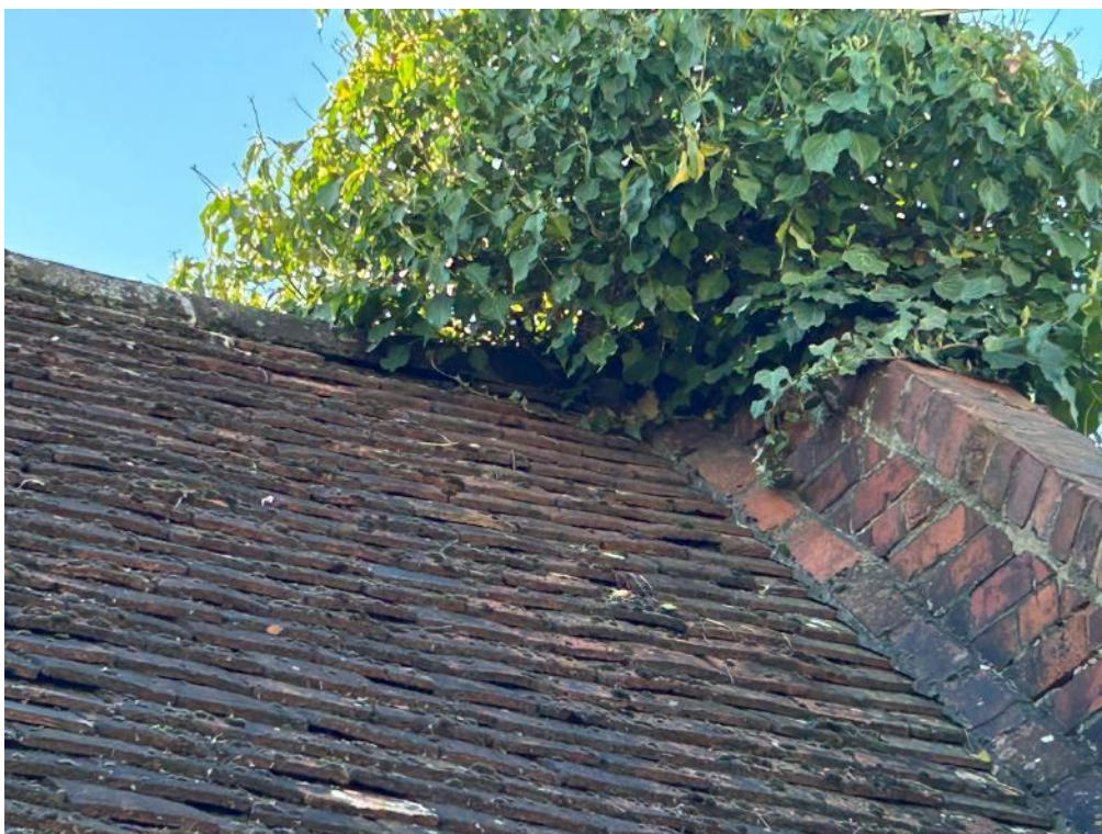
Photograph 41: Barn, missing and lifted tiles and gaps at ridge, northern gable end
