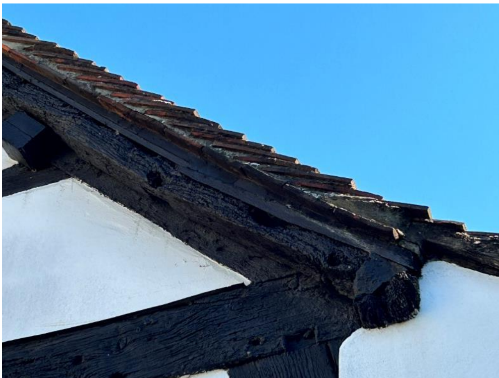
Photograph 36: Main pub, gaps/damage to wooden eaves, northern elevation
