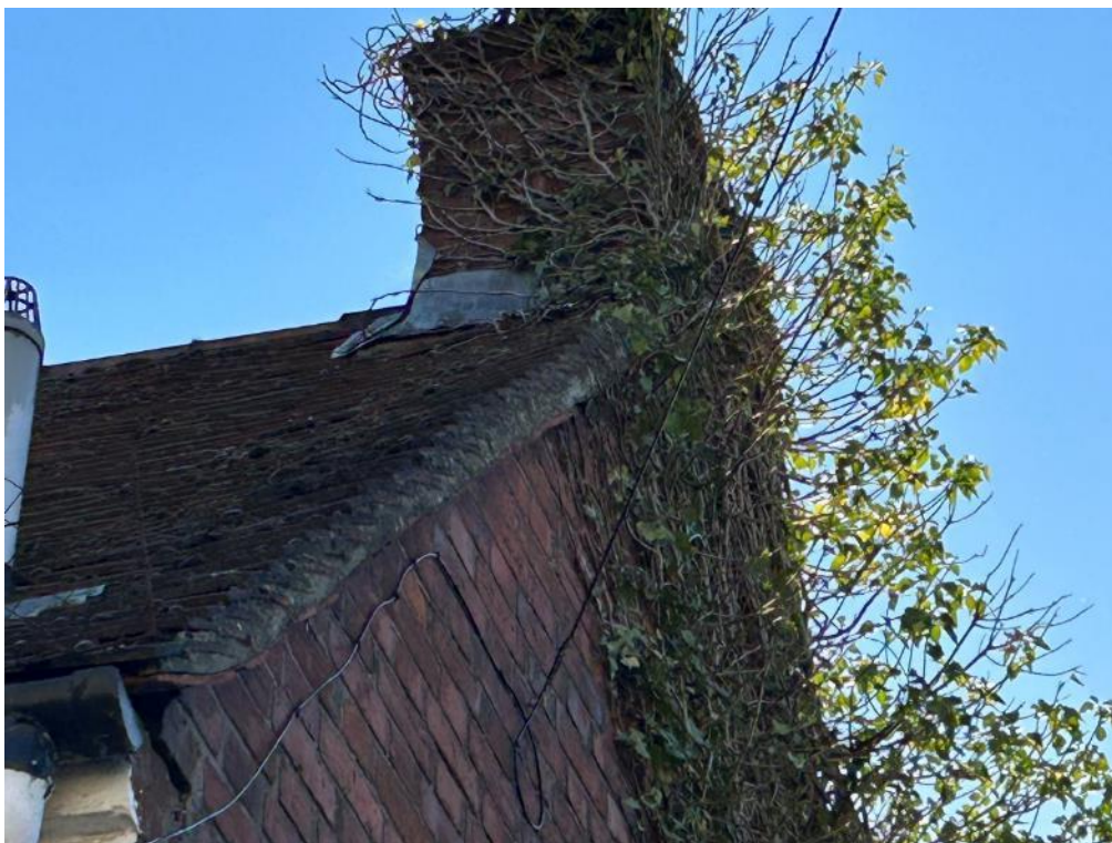
Photograph 38: Main Pub, eaves overhanging Barn, lifted lead flashing and ivy lattice
