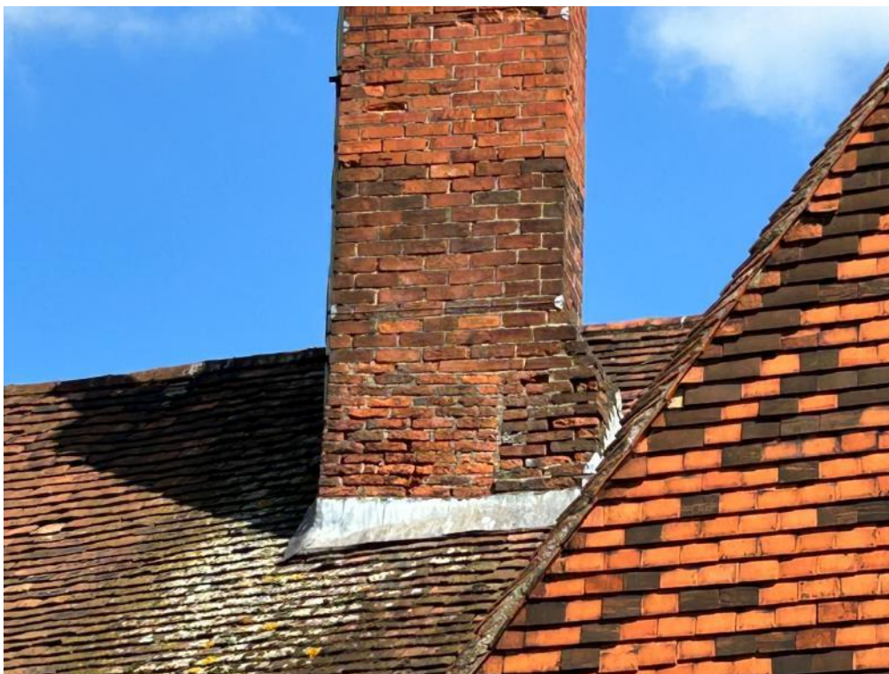
Photograph 34: Main Pub, lifted flashing at chimney stack and missing mortar
