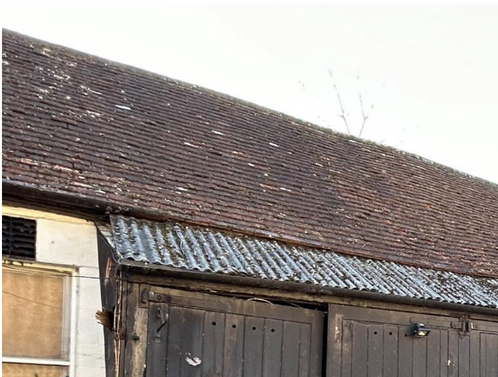
Photograph 40: Barn, missing and lifted tiles, eastern elevation
