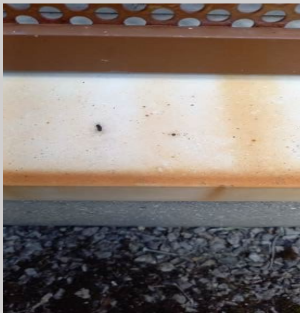
Photograph 23: Bat dropping on exterior of Building 3
