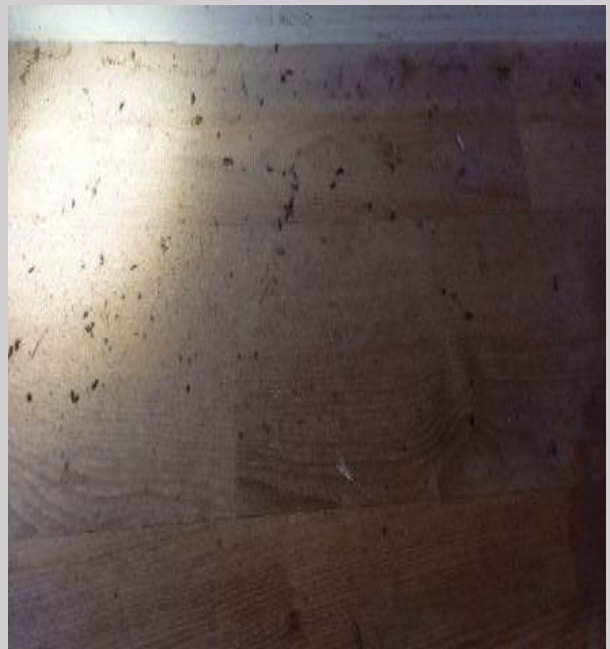
Photograph 24: Bat droppings in interior of Building 3
