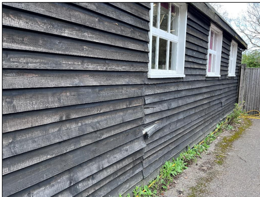
Photograph 1: weather damaged cladding beginning to lift.
