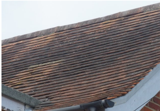
3. Occasionally lifted tiles near front gable (southeast elevation).
