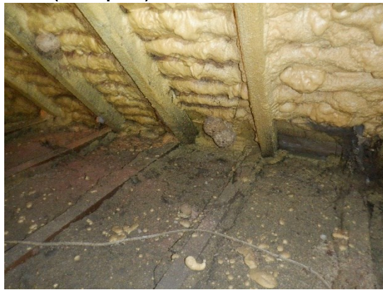
22. Small wasp nests present in eaves (roof space).
