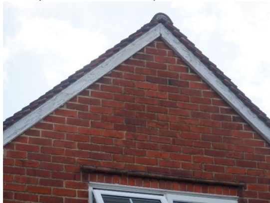
12. Narrow gaps behind gable barge boards (rear elevation).
