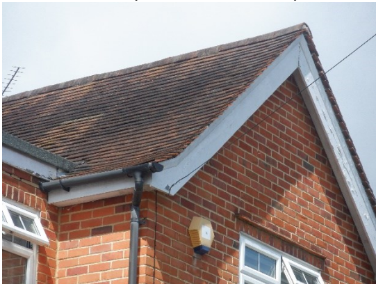
11. Narrow gaps behind gable fascias (front elevation).
