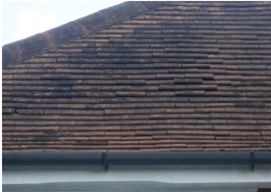
4. Occasionally lifted tiles (rear elevation).
