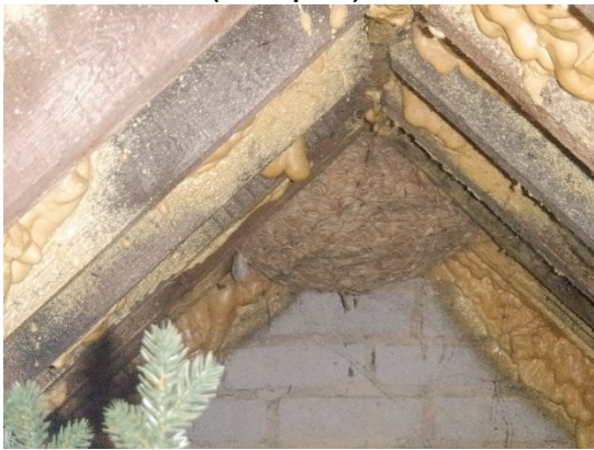
21. Large wasp nest at rear gable end (roof space).
