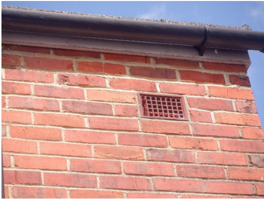
9. Slight gaps behind fascias on flat roof extension (southeast elevation).
