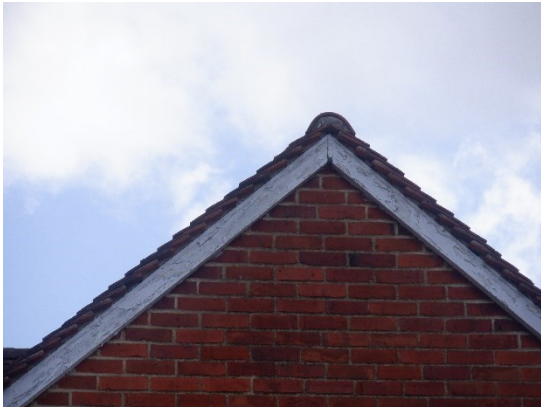
7. Gap in verge mortar at rear gable apex (rear elevation).
