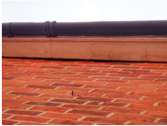
8. Large gap behind soffit box (northwest elevation).
