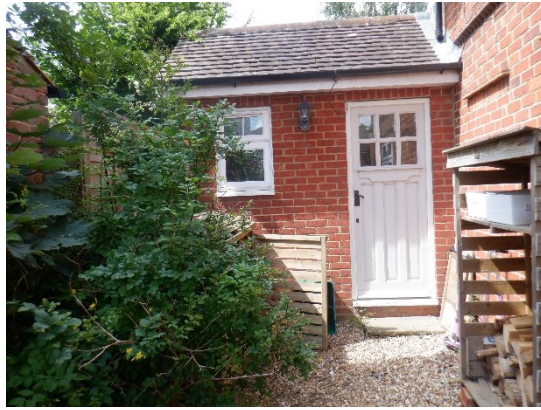
14. Slightly lifted roof tiles on garage (front elevation).
