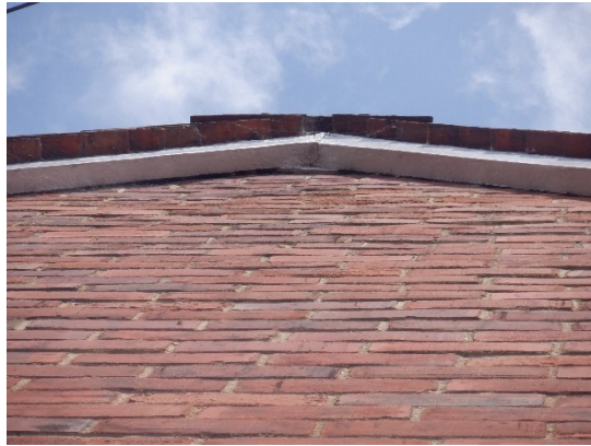
10. Large gaps behind gable fascias (southeast elevation).
