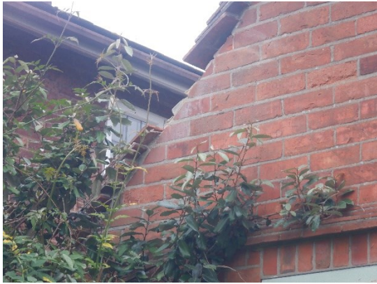
13. Missing tiles on garage roof.
