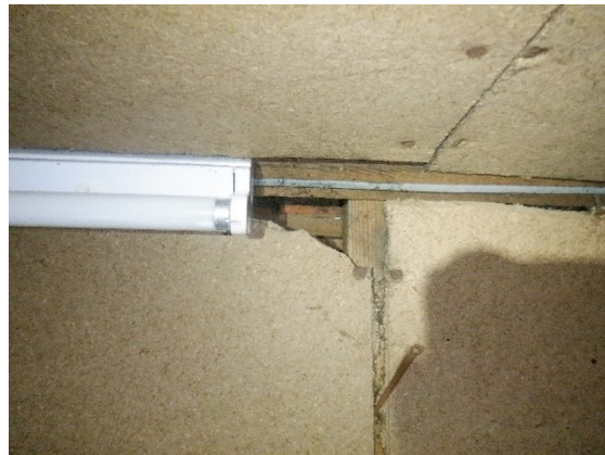
18. Occasional gaps in boarding.
