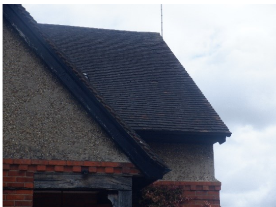
5. Roof tiles with occasionally lifted tiles.
