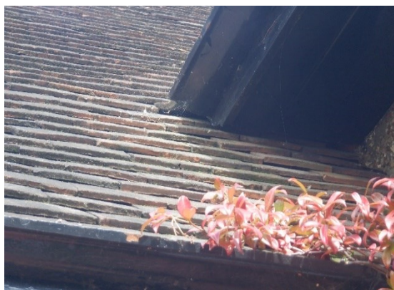
6. Roof tiles with occasionally lifted tiles.
