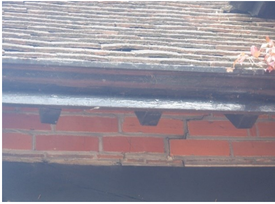
7. Roof tiles with occasionally lifted tiles.
