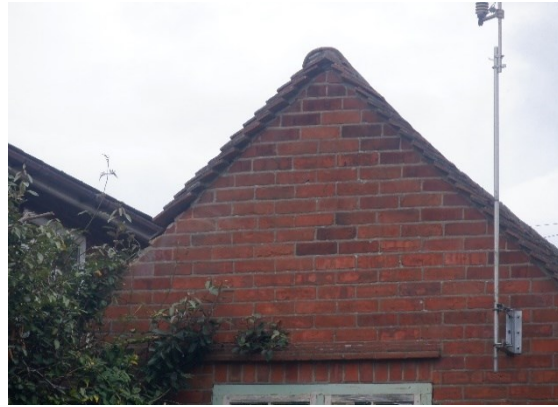
14. Missing mortar on verges.
