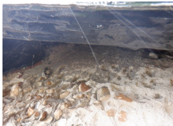
12. Gap behind soffit on porch investigated thoroughly.
