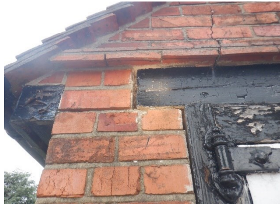
16. Gaps around timber door frame.
