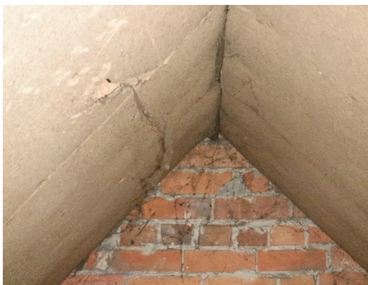
21. Gap at apex of blockwork gable, heavily cobwebbed.
