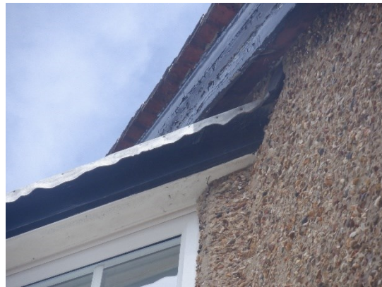
10. Gaps behind the lead flashings
