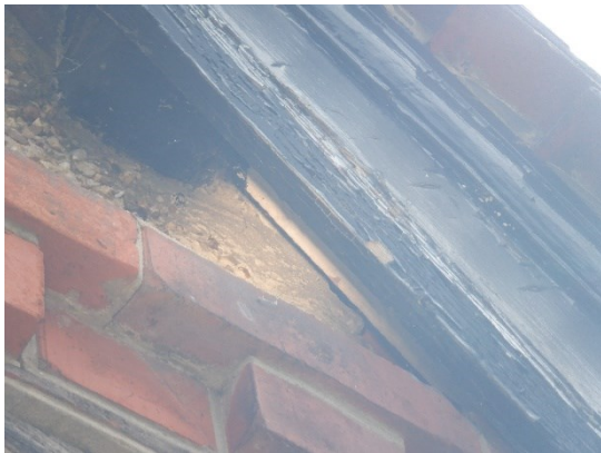
9. Gap behind front gable barge board.
