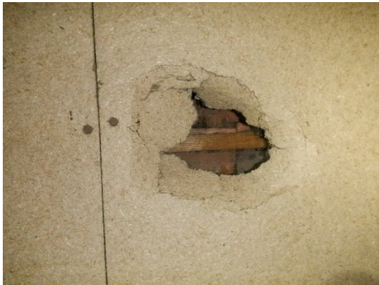
19. Occasional gaps in boarding.
