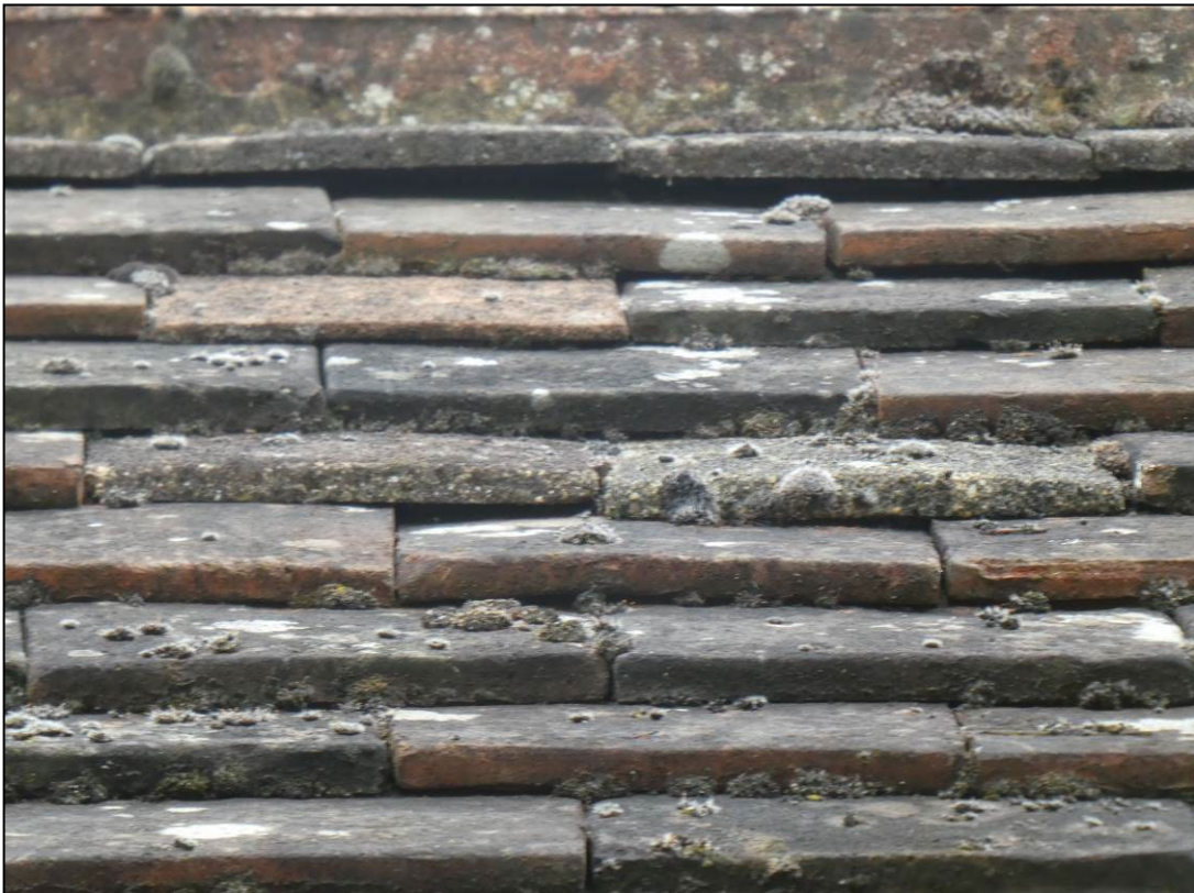
Figure 5. Example of lifted roof tiles. 46 Grosvenor Road, Caversham. 12.09.23
