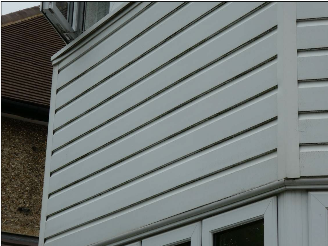
Figure 9. PVC cladding on front of building. 46 Grosvenor Road, Caversham. 12.09.23
