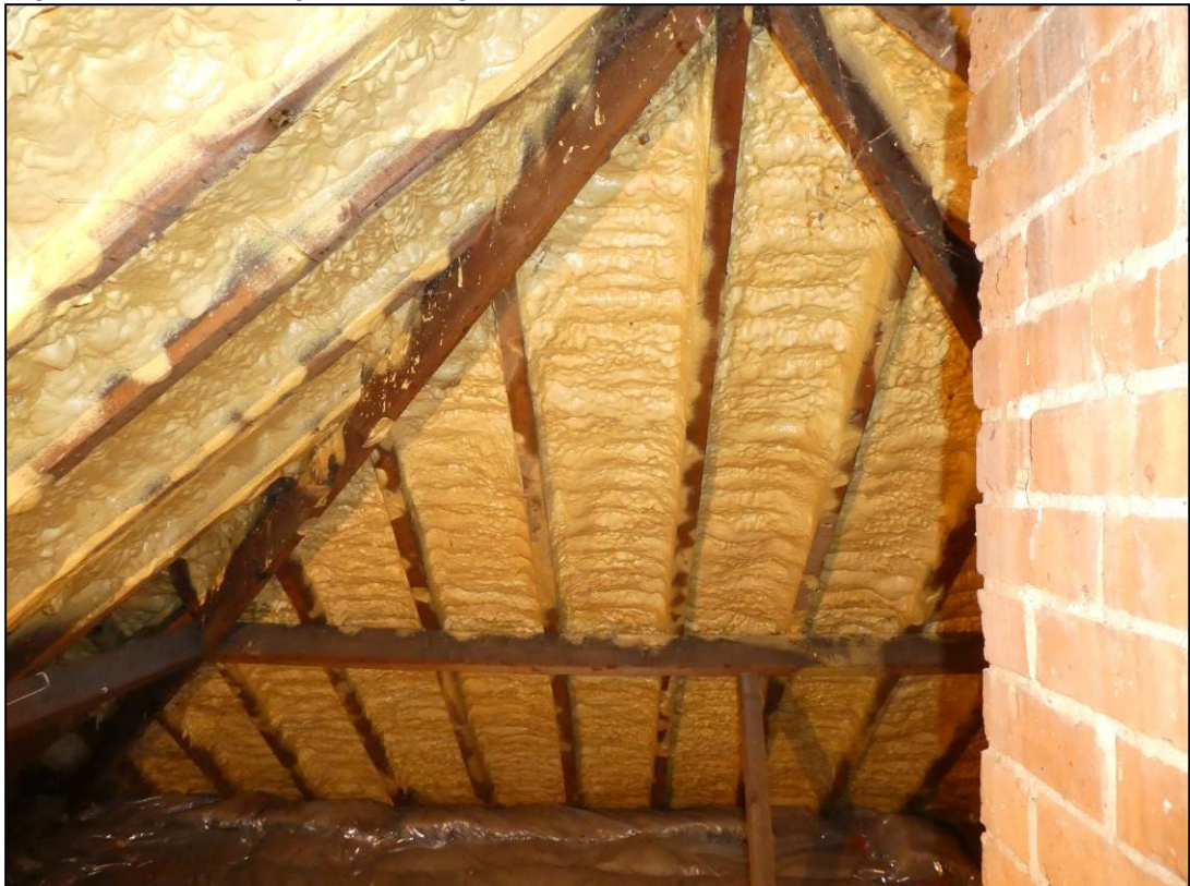
Figure 16. Expanding foam lining roof tiles. 46 Grosvenor Road, Caversham. 12.09.23
