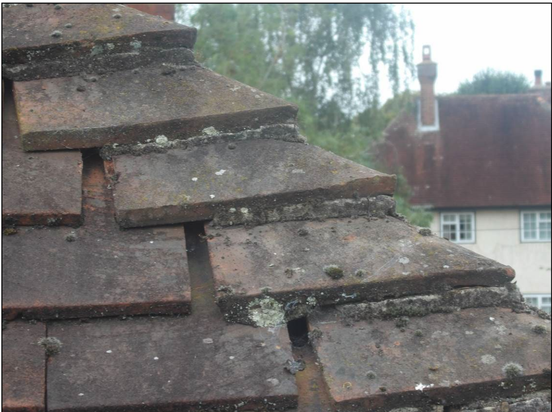
Figure 7. Gaps between roof and hip tiles. 46 Grosvenor Road, Caversham. 12.09.23
