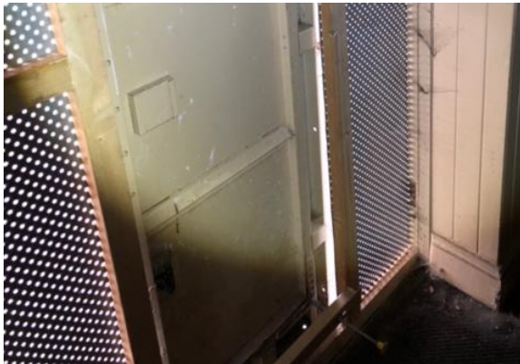
Photo 13: The door leading to the carpark/garden – with 3-5 cm gaps. This room leads to the uninspected roof space and the damaged ceiling.
