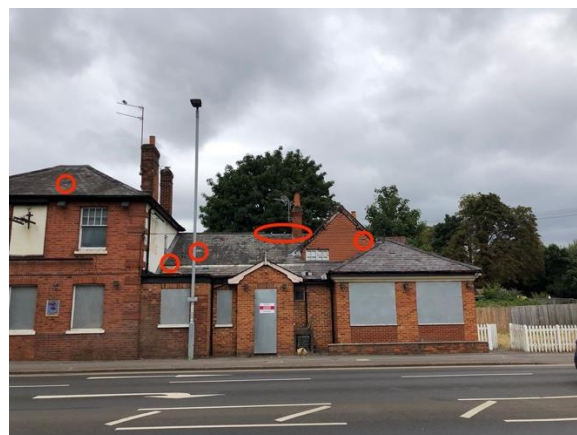
Photo 20: Location of several missing slates on the front (south-facing) of the building.
