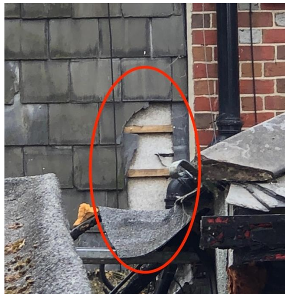
Photo 18: Missing / damaged slates (wall) on the upper floor with the flat roof (north facing).
