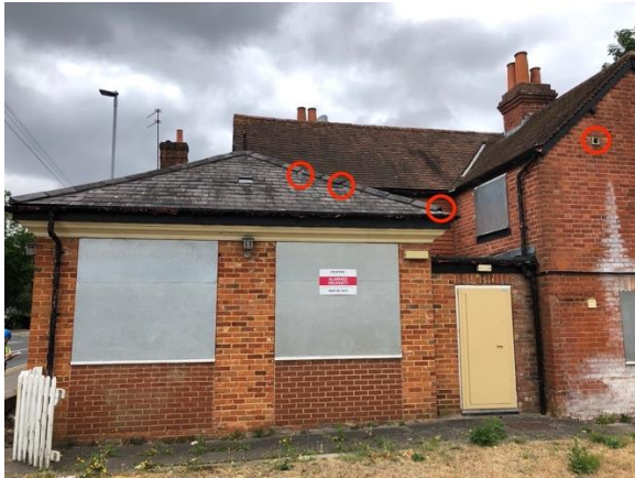
Photo 21: Potential features on the eastern side of the building – slipped ridge tiles and a hole in the wall.
