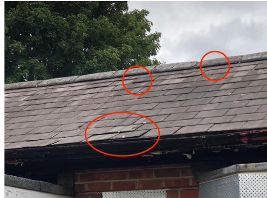
Photo 14: Slipped tiles and missing pointing on the roof.
