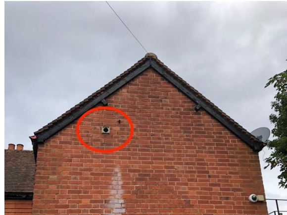
Photo 22: The missing ventilation cover.
