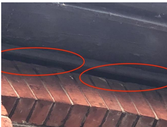
Photo 19: Gaps between the brickwork and soffit on the front left (upper) wall/window – road-facing.
