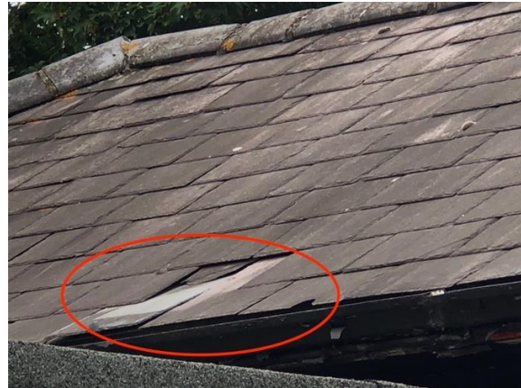
Photo 16: Some of the missing tiles on the north-facing roof.
