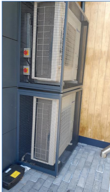
Fig 1. HVAC Condensing Unit to the rear of Starbucks. Photo taken by case officer on 21/06/2023
