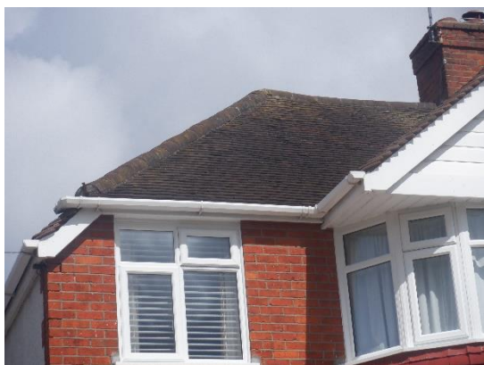
5. Ridge and hip tile mortar mostly intact throughout.
