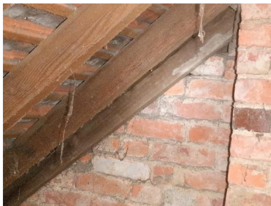
14. Small gaps in party-wall brick gable end behind rafters.
