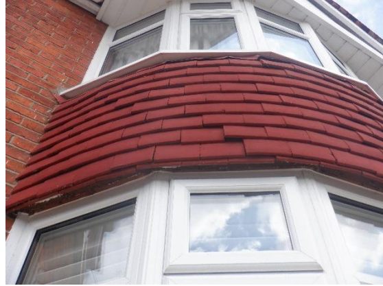
8. Occasional gaps behind hanging tiles.
