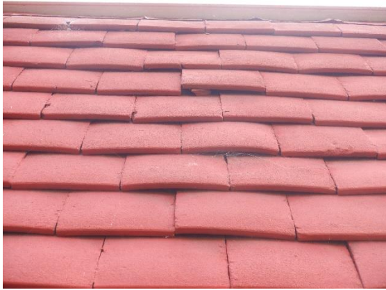
7. Occasional gaps behind hanging tiles.
