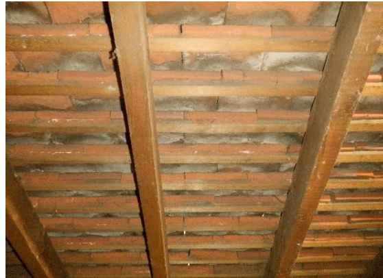
10. Roof unlined and draughty with daylight visible.
