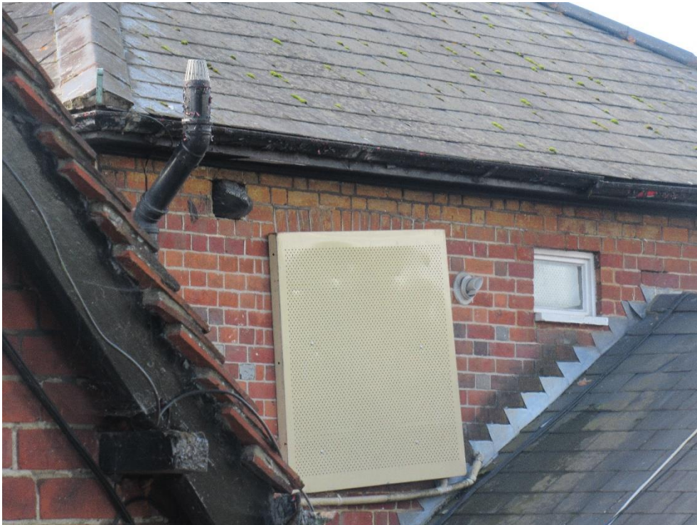
Plate 24 – North elevation of the main building showing infilled opening and change to the brickwork to the upper courses
