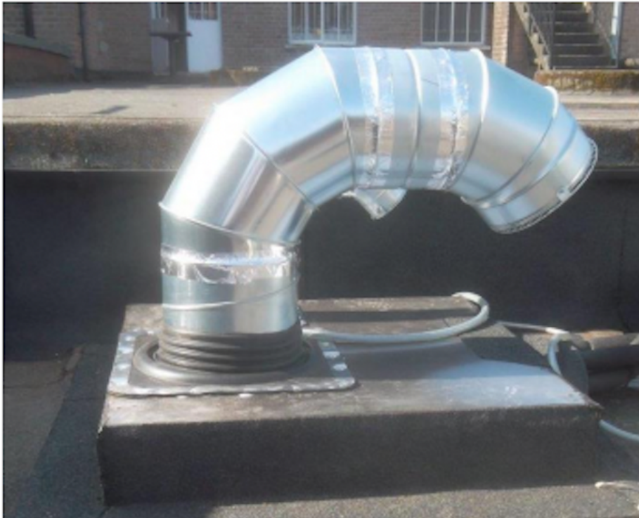
Fig.5 – Kitchen Extract System Roof Cowl
