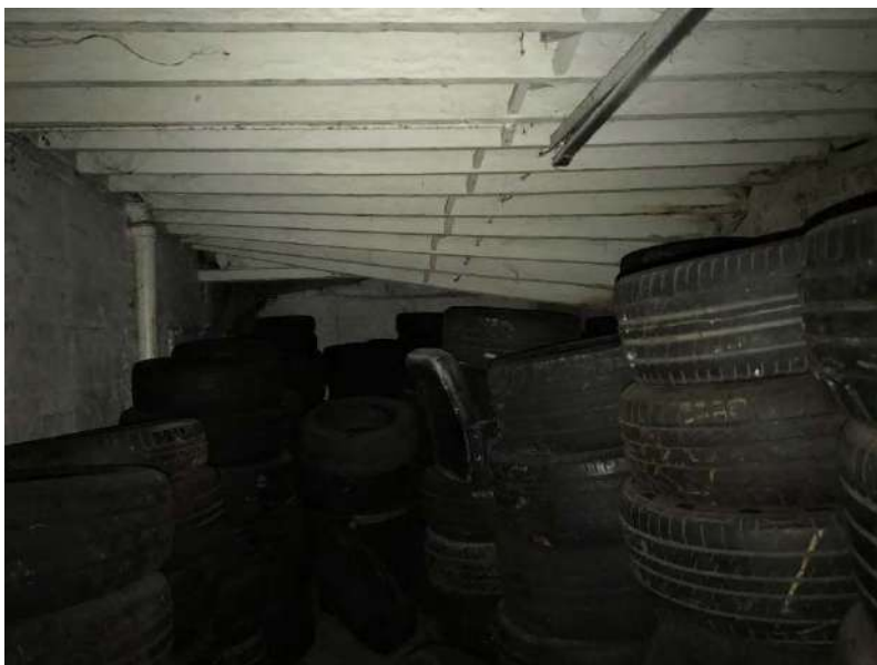
Plate 40: Collapsed floor in the southern end of Building 3.
