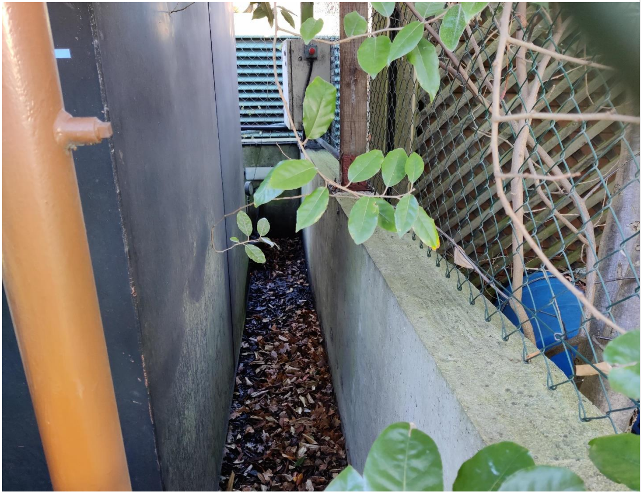
Plate 5 - Inside AST cage, gauge noted associated with the tank. Water noted on the floor.
