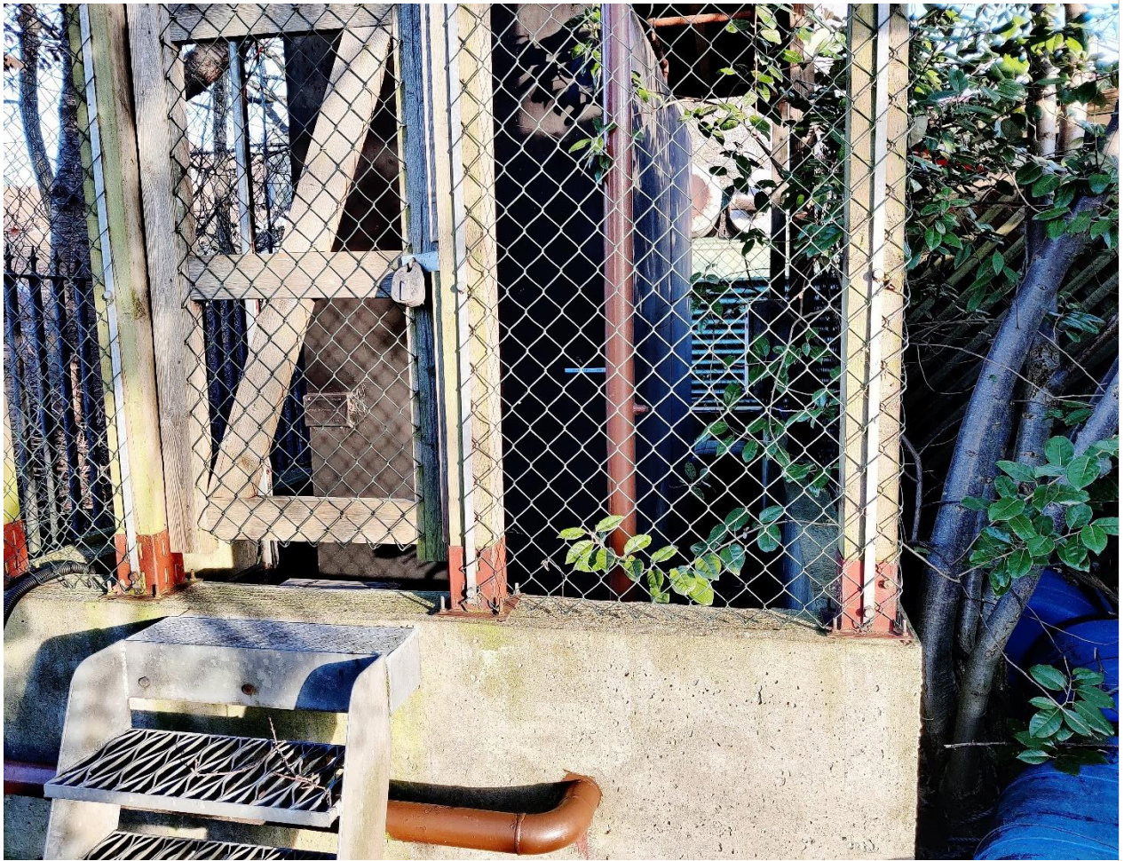
Plate 3 - Steel banded AST within concrete and wooden building.
