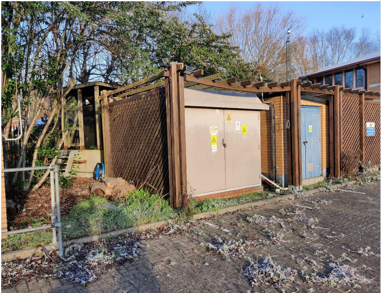
Plate 1 - Electrical substation and above ground storage tank (AST) on western portion of the Site.
