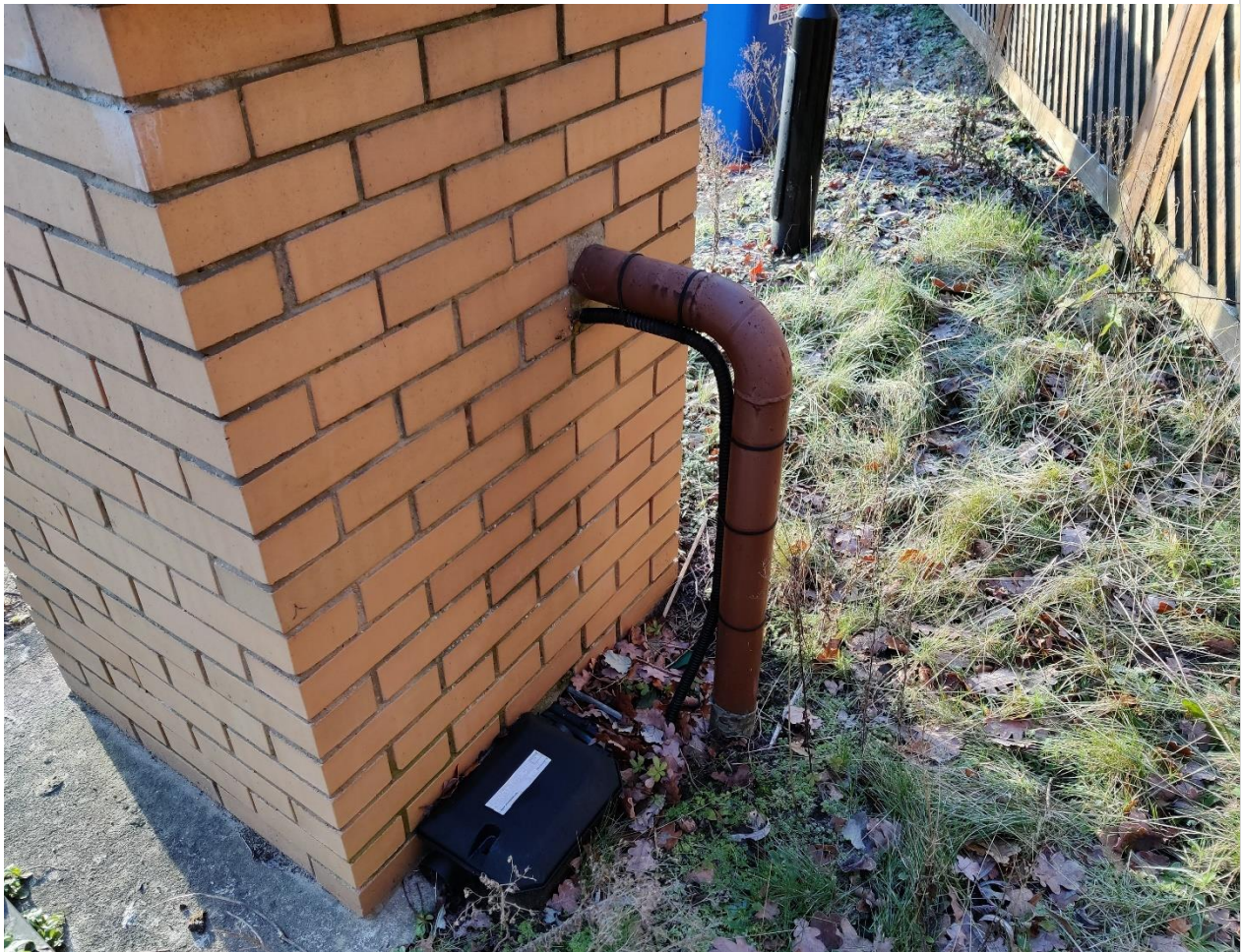
Plate 7 - Pipe/ducting on the back of the filling point going underground.
