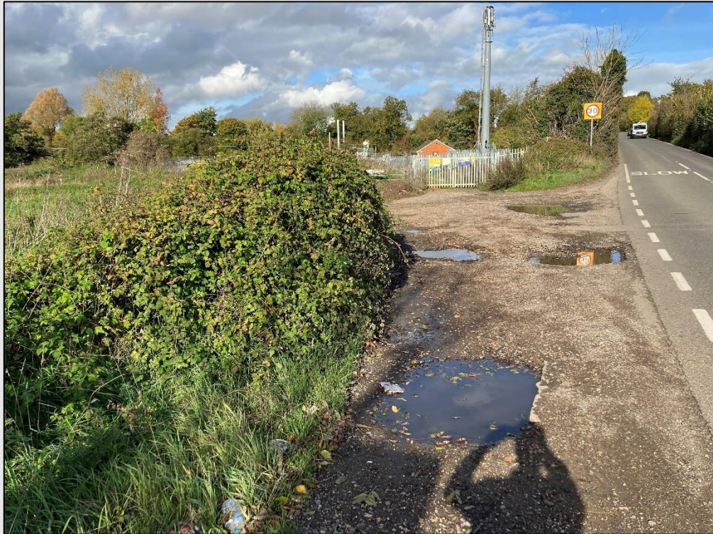
Figure 6. Hard standing tarmacked road access in poor condition.
