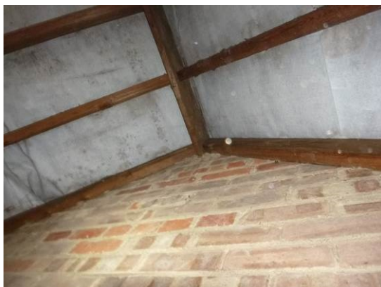
13. Gaps behind rafters at gable end (roof void).
