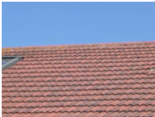
4. Securely mortared ridge tiles (rear elevation).
