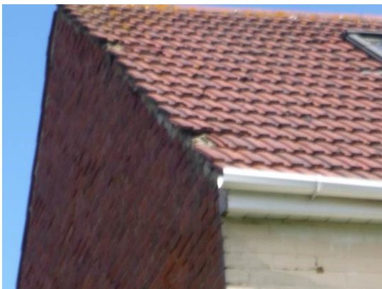
3. Couple of missing verge tiles (rear elevation).
