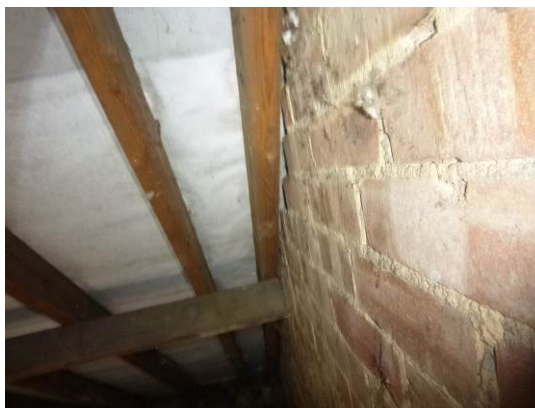
14. Gaps behind rafters at gable end (roof void).
