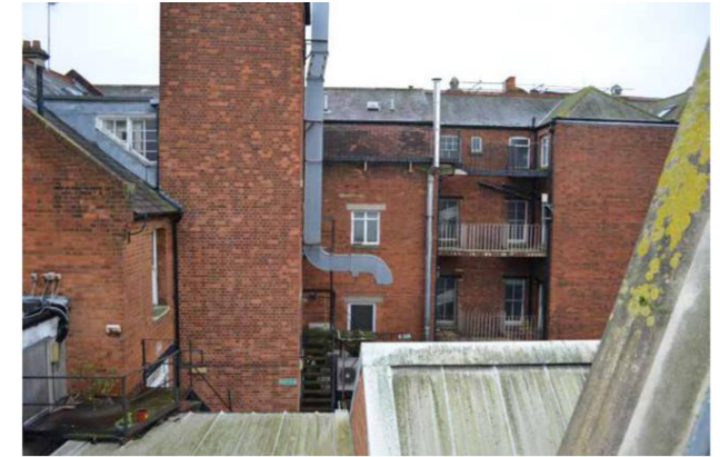
Figure 4.6 Poor quality rear elevations of the site
