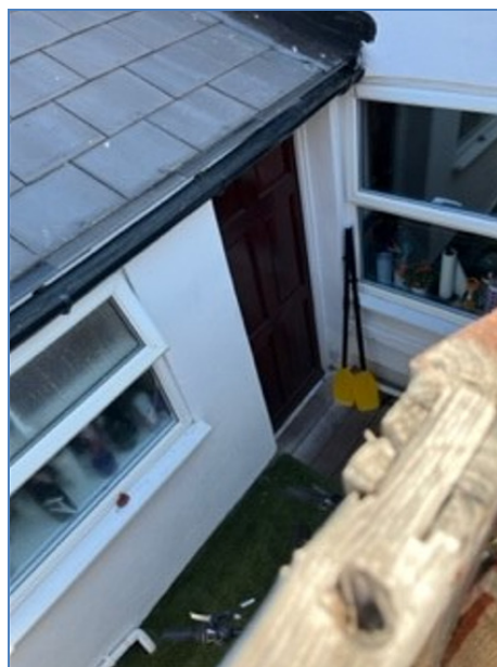
Fig 3. Bathroom and Kitchen to 80 Mount Pleasant. Photos provided by Agent on 31/07/2022.
