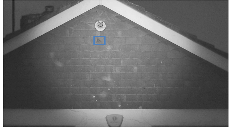
2. Common pipistrelle emerging from roost through missing hanging tile (highlighted in blue) at 21:57 (Survey location 1).
