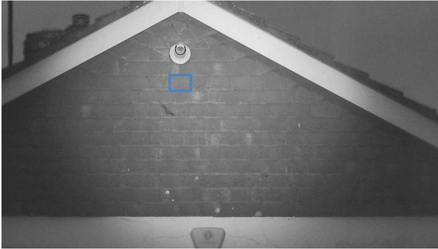
1. Common pipistrelle entering roost through missing hanging tile (highlighted in blue) at 21:53 (Survey location 1).
