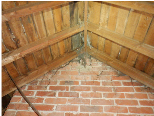
15. Cobwebbed brickwork party wall (roof void).
