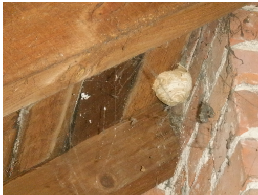
16. Cobwebbed chimney with small wasp nest on brickwork (roof void).
