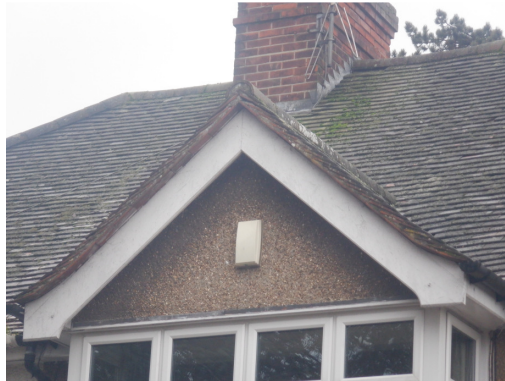
8. Crack in verge mortar on gable (front elevation).
