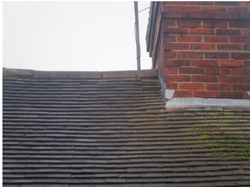
7. Missing mortar below ridge tile by chimney (rear elevation).
