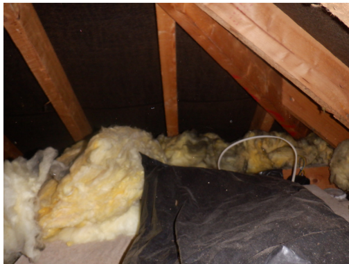
18. Eaves blocked by fibreglass insulation in rear hipped roof (roof void).
