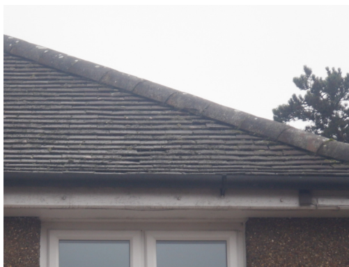
6. Gaps below hip tiles (front elevation).
