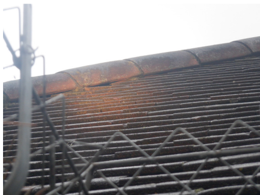
5. Gaps below hip tiles (rear elevation).
