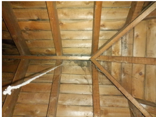
12. Cobwebbed ridge (roof void).
