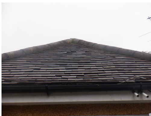
4. Lifted and uneven roof tiles (rear elevation).
