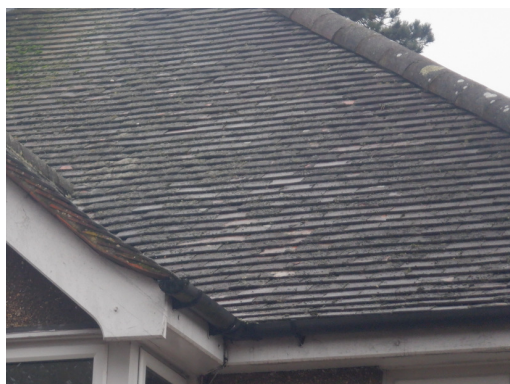
3. Occasionally lifted roof tiles (front elevation).
