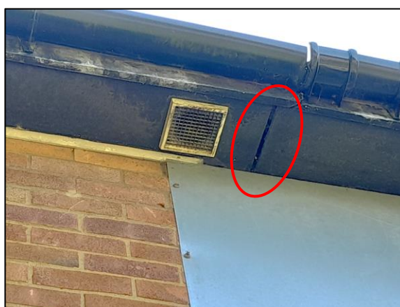
Photo 16 Gap to soffit
