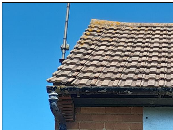
Photo 13 Lifting to tiles on eastern edge of south roof face
