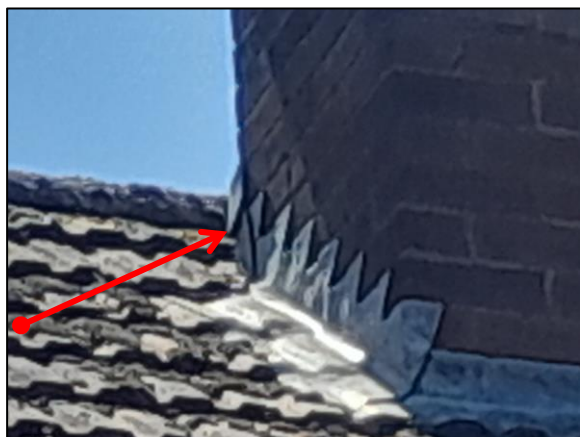
Photo 19 Lifted flashing behind chimney
