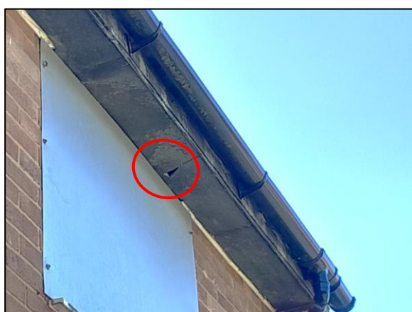
Photo 15 Soffit to rear well sealed, but damage present
