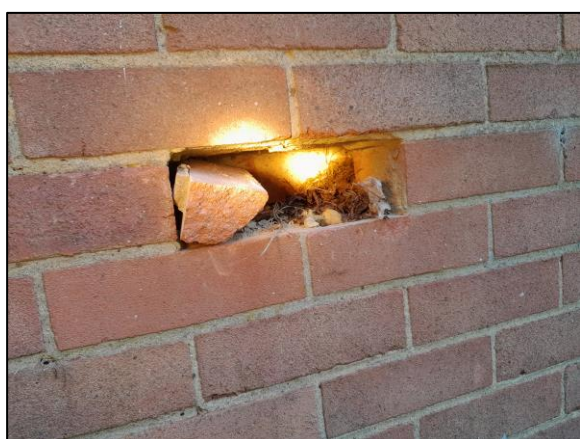
Photo 17 Missing brick with bird nest and potential bat access to wall cavity
