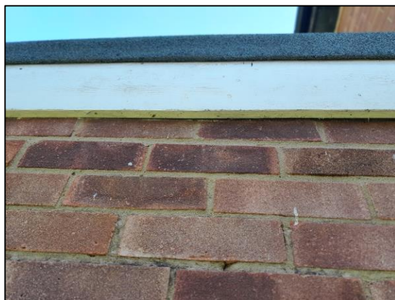
Photo 20 Flat roof fascia tight to wall
