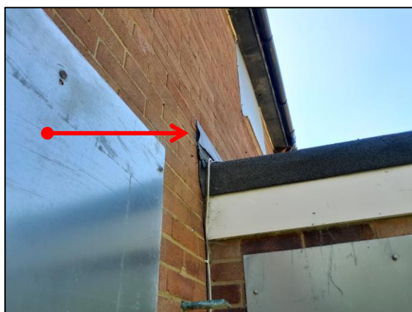
Photo 21 Gap to flashing to rear flat roof extension
