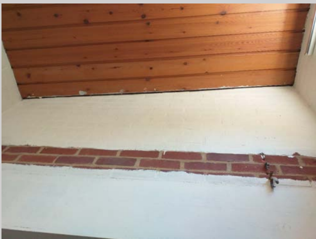
Photograph 15: Gap between wall and wooden ceiling, droppings at location D were found below this feature.
