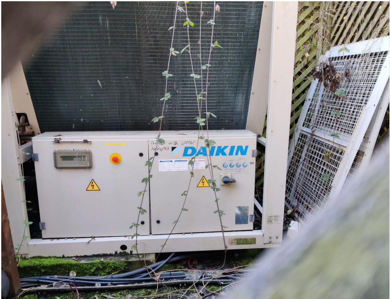
Plate 8 - Air conditioning units on north-eastern part of the Site.
