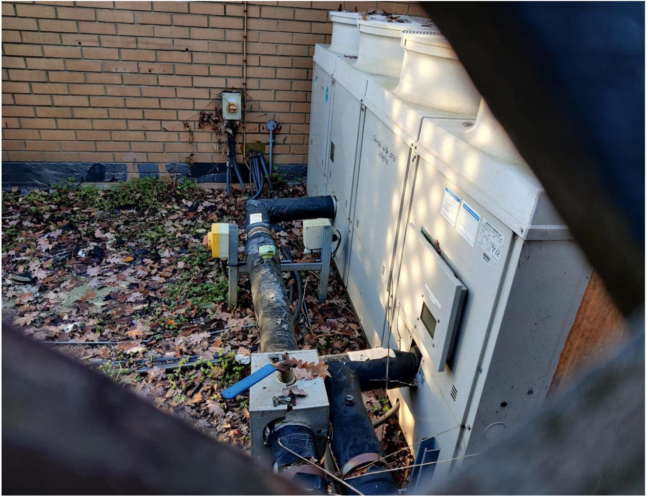
Plate 9 - Air conditioning units on western part of the Site.
